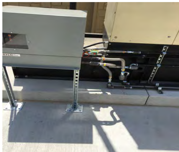
GENSET PUMP AND PIPING
